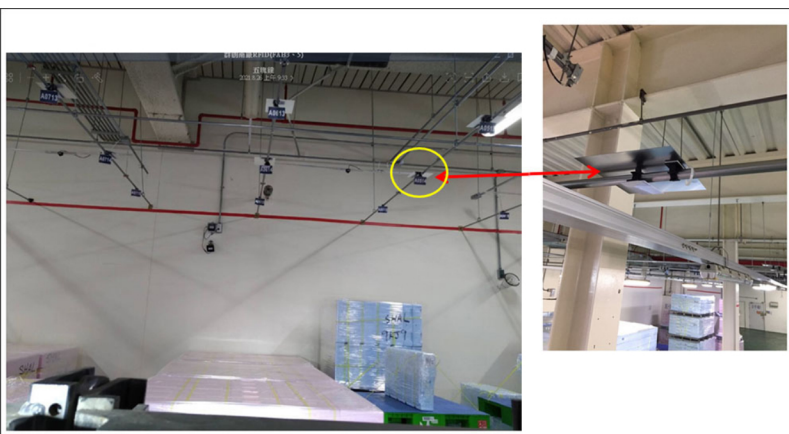
A position tag is located on the ceiling.
